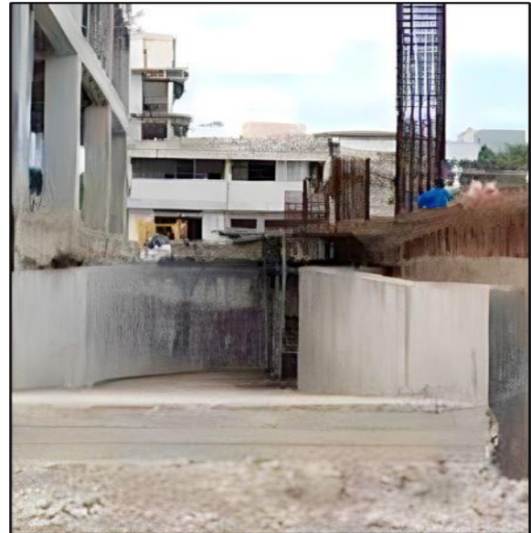
Gambar 5. Kegagalan Temporary Structure Perancah Sumber : Pre Construction Meeting Proyek Bandung Advanced Science and Creative Engineering Space (BASICS) (Paket 3)
